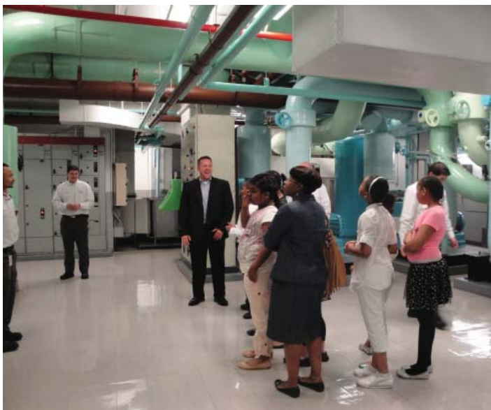
Chief Building Engineer at Hogan Lovells, Jim Ferranti, explains to Kimball Elementary School students how he and his staff keep all the systems in the law firm's building working properly.
