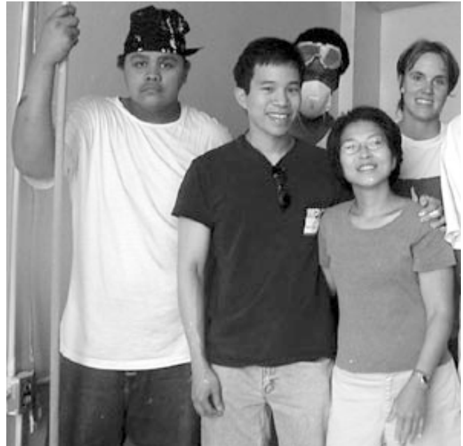
Clinic office renovation crew. L/R, First row: Cardozo student; Robert Wone, Covington & Burling attorney; Katherine Wone. Second row: Cardozo student; Kerry Sylvia, Cardozo teacher.
